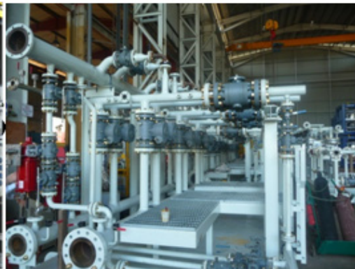
PLATFORM PRODUCTION MANIFOLD
